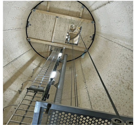
The wooden parts of the turbine tower are glued together on site
